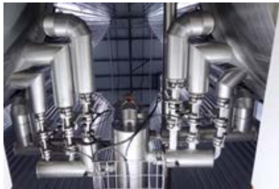
Glycol valve station
